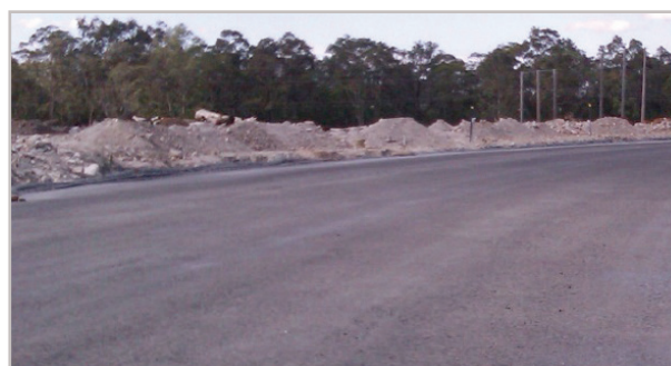
Figure 5.4 - Heavily Bound Pavement.
