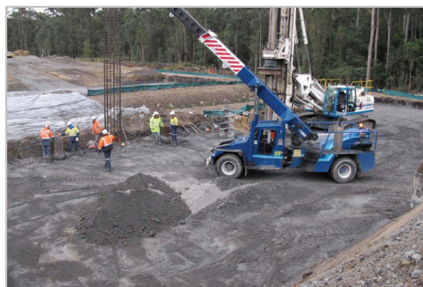
Figure 5.5 - Hunter Expressway piling works at bridge BW13 on a layer of stabilized road base.
